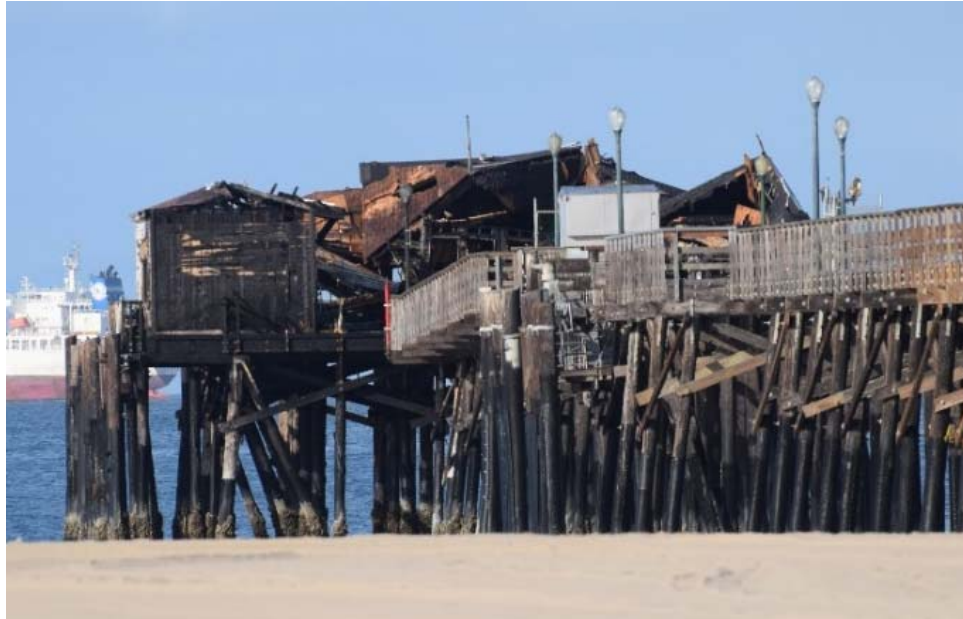
Figure 10. Seal Beach Pier May 2016 Fire Damage
